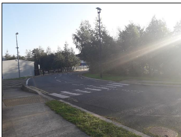
Figure 3.18 Faded road marking along main access road towards Piper's Hill College
